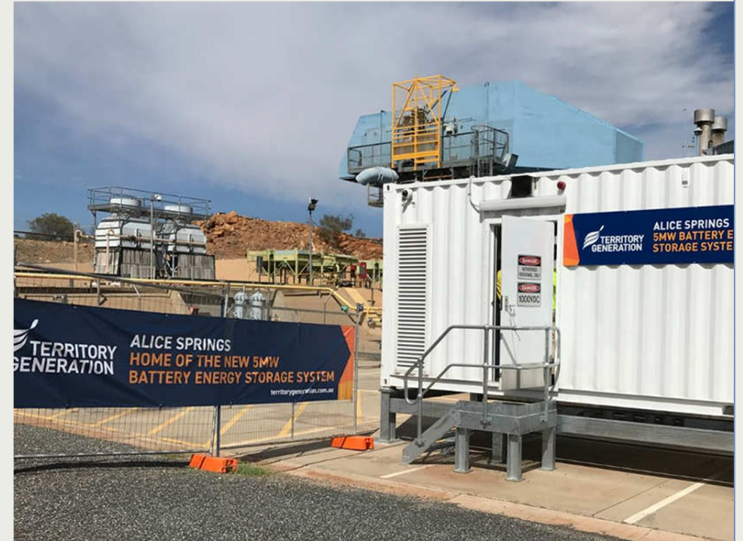
Brewer Estate battery and gas fired power plant... enabling 43% solar in Alice Springs 50% by 2030
